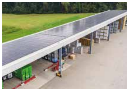
Photovoltaic system on flat roof of warehouse
